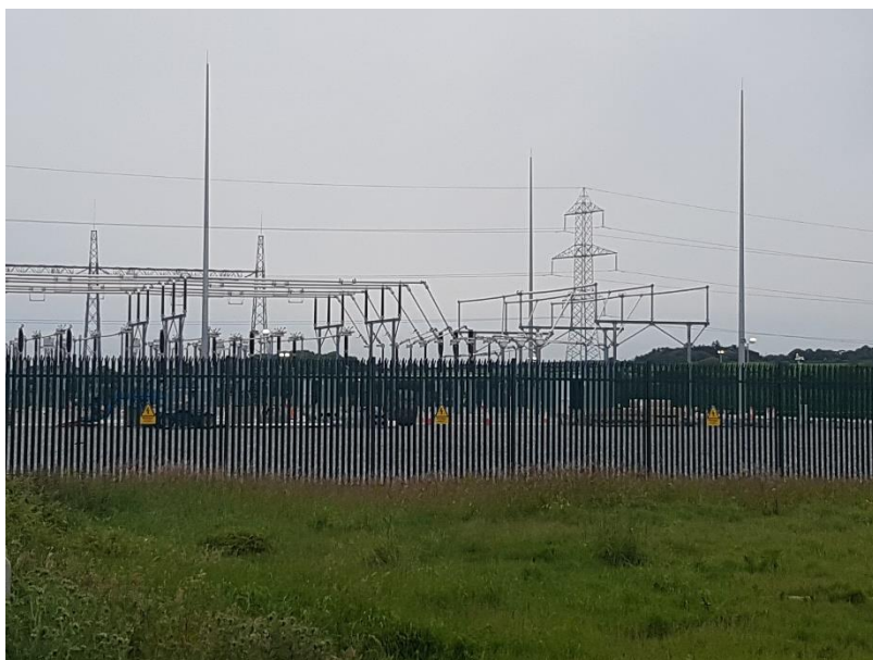
Figure A2.2.1: Typical Example of 220 kV Substation
